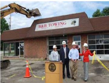
County Councilman, John Schmidt (District 2) with Summit County Director of Development Connie Kraus(left), County Executive Russ Pry and Cuyahoga Falls Community Development Director, Susan Truby at Demolition Ceremony for B&B Towing.
